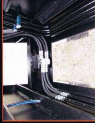
Neat, Professional Mounting of Tubes, Hoses, and Valves
